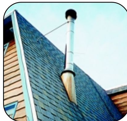
Every chimney and stovepipe must be covered with no larger than \frac{5}{8} -inch nonflammable screen.
