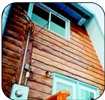
Roof eaves should be enclosed with fire-resistant materials and vents screened with \frac{1}{4} -inch nonflammable mesh screen.
