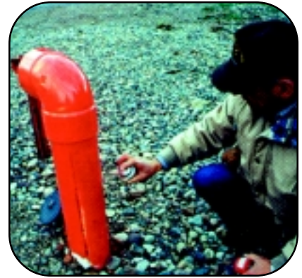
You can install a dry hydrant to improve accessibility to your water source.
